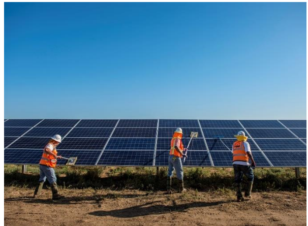
© Dave Lauridsen | Workers clean solar panels for maximum efficiency at the power solar facility in Lancaster, CA.
